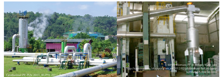
Geothermal PP, PLN 2011, RUPTL 2011-2020, page 49
