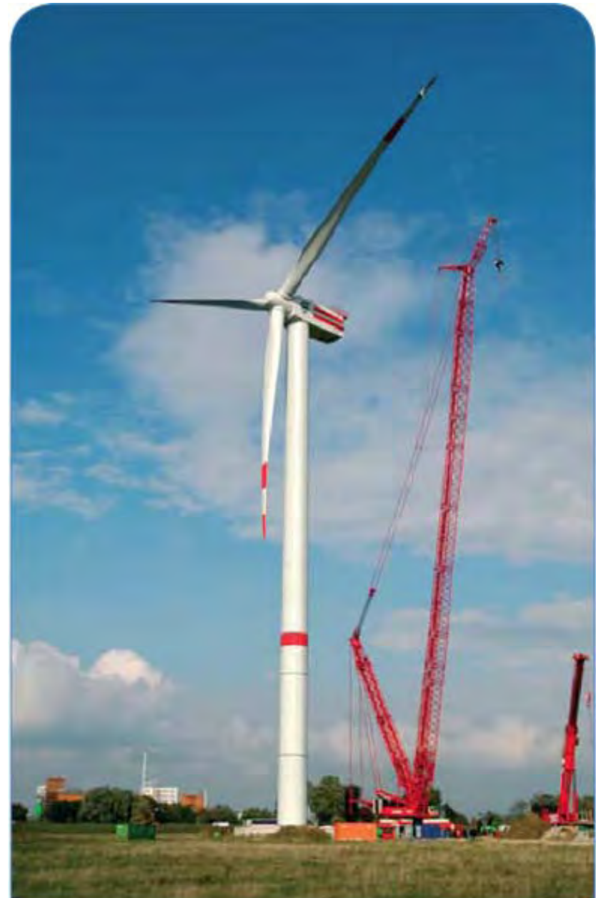
Prototype of RePower 5 MW wind turbine installed at Brunsbüttel, Germany. With a rotor diameter of 126 m, it is the largest wind turbine ever built.
