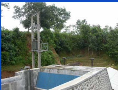
TRASH RACK Manual-Automatic Cleaning
